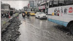
SUMPY RIDER: A damaged service road near Vyttila Junction
