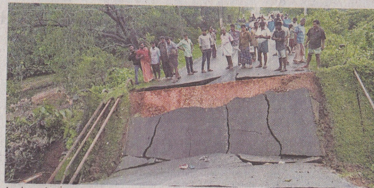
A culvert that caved in near Kothamangalam on Wednesday. ■ SPECIAL ARRANGEMENT
