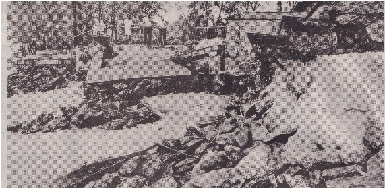
A compound wall built close to the sea destroyed in the heavy rain that lashed Kozhikode district during the past couple of days. A scene from Kappad beach | TP SOORAJ
