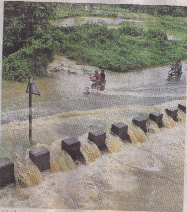
Vehicles moving on the Kazhachaparambu-Kannadi road in Palakkad that was flooded in heavy rain on Tuesday. Three days of torrential rain flooded roads and inundated farmlands in many parts of the State. *K.K.MUSTAFAH
