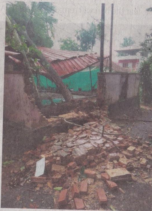
As per an assessment, 53 houses in Eloor suffered damage while three were fully destroyed in strong winds on Monday.
