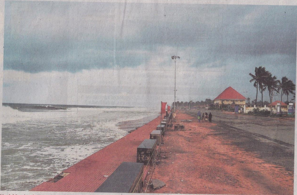
Vanishing land: Shanghumughom beach in Thiruvananthapuram wears a deserted look as erosion has taken away much of the beach and a part of the road. Domestic tourists usually frequent the beach in large numbers. ■ S. GOPAKUMAR
