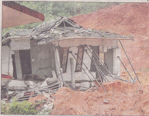
The house collapsed due to a landslide near Peringavu in Malappuram
