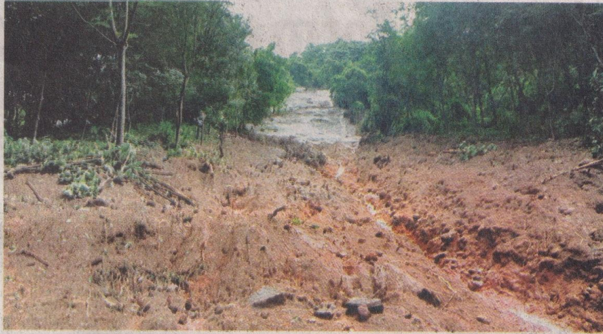
The stretch at Ambalappara on Vazhachal-Malakkappara Road, which caved in following heavy rain on Wednesday
