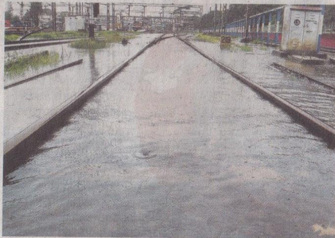
The flooded rail track near the South railway station. ■ H. VIBHU
